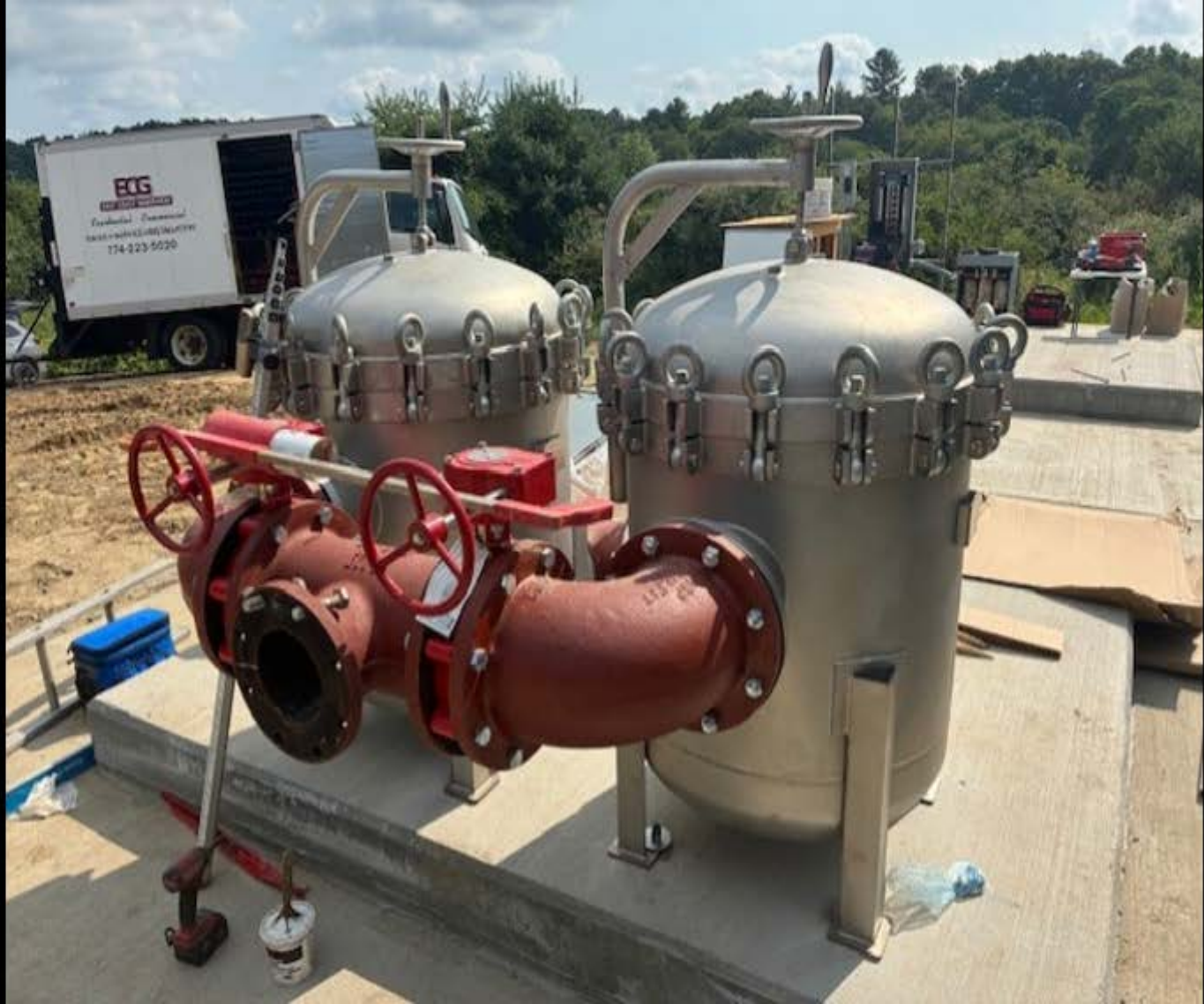
Bag filters mounted on pedestals, ready for connection.
